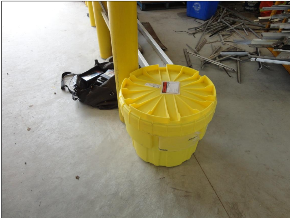
Figure 2: Battery spill kit accessible on site.
