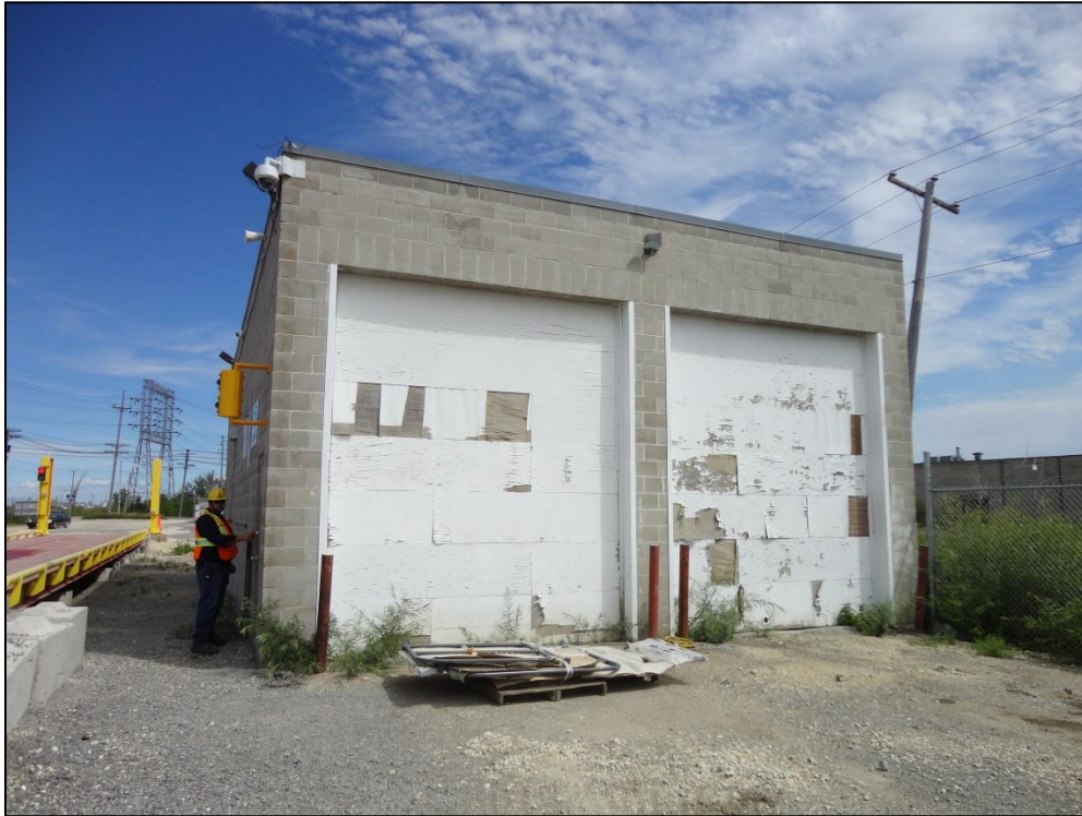
Figure 1: Two sliding doors on the exterior of the battery storage building used for loading. Due to the age of the sliding doors, they are slated to be replaced shortly.
